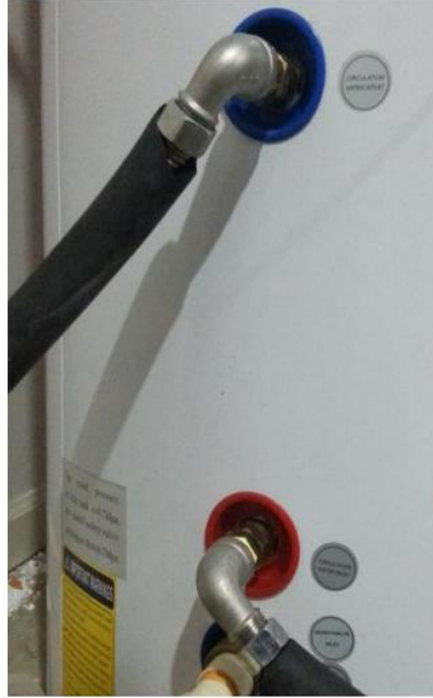
Elbows used on Solar Loop Connections to Tank to Prevent Thermo Siphon Effects
