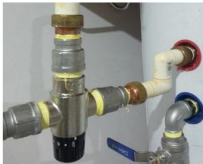
1" Thermostatic Mixing Valve Connected to Hot Water Outlet and Cold Water Inlet
